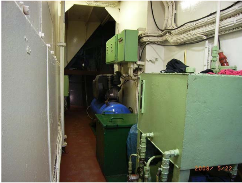
Photo 1. Confined entrance room with operating panels. The hold entrance door can be seen as the dark green box in the centre of picture
